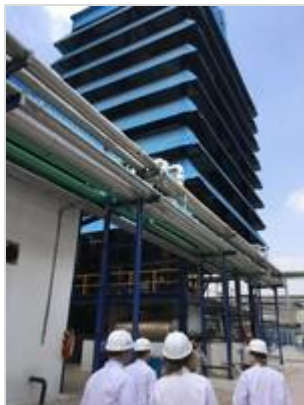
Solvent tower at Sami Lab's Kunigal facility.
